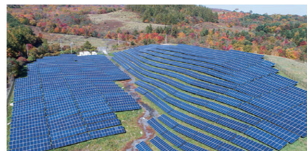
Kamaishi Naranokidaira Solar Plant
