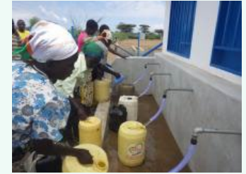
Republic of Kenya – The Project for Rural Water Supply in Baringo County
