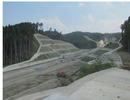
▲ Shin-Meishin Expressway while under construction (Shin-Yokkaichi Junction to Komono) Opened in March of 2019
